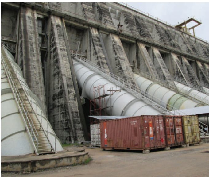
Inga 1 and Inga 2 built in the 1972 and 1982, respectively, are in a rundown state and cannot meet the energy needs of the DRC.
